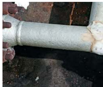
Corrosion Under Insulation
